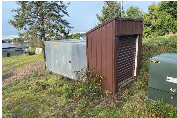
Figure 4-18 | Lower Blackstone Pump Station
