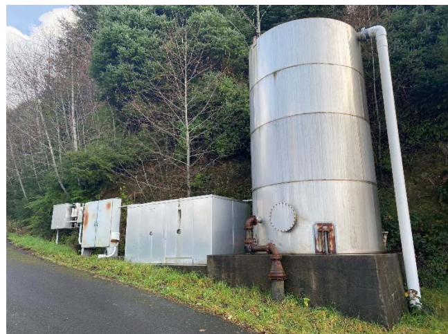
Figure 4-14 | 10,000 Gallon Middle Blackstone Reservoir & Pump Station
