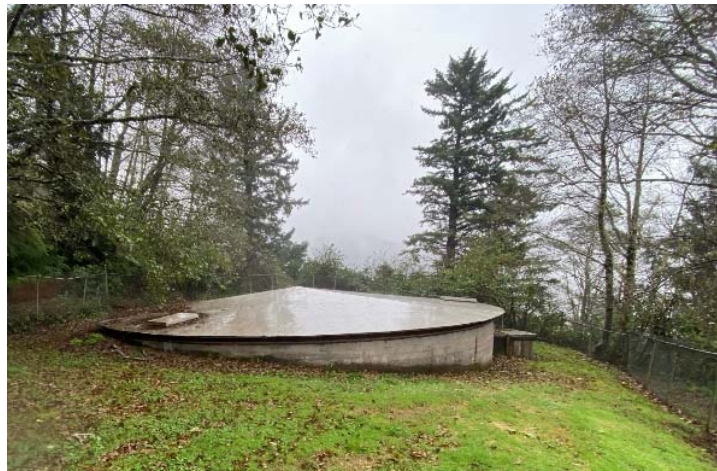
Figure 4-11 | Lower Radar Road Reservoir
