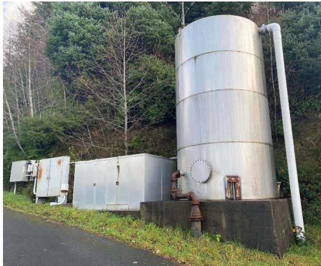
Figure 4-19 | Middle Blackstone Pump Station & Reservoir
