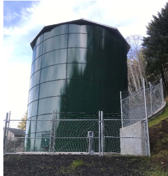
Figure 4-13 | 250,000 Gallon South Reservoir
