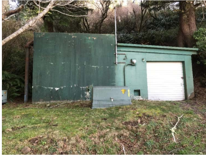
Figure 4-12 | 10,000 Gallon Horizon Hill Reservoir & Pump Station
