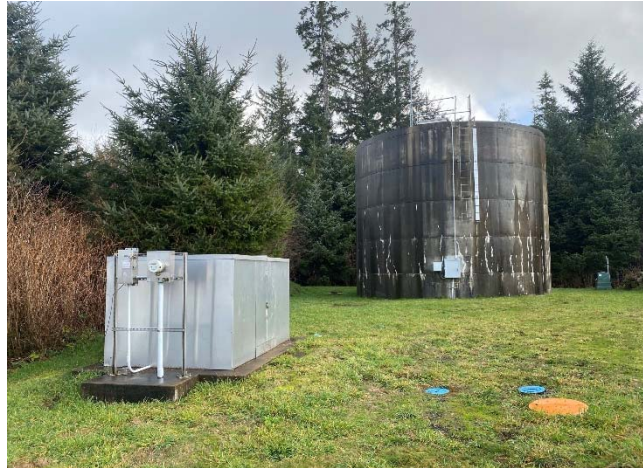
Figure 4-15 | 120,000 Gallon Upper Blackstone Reservoir and Pump Station
