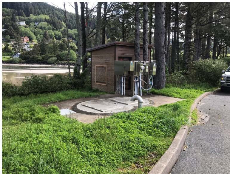
Figure 4-6 Parkside Pump Station
