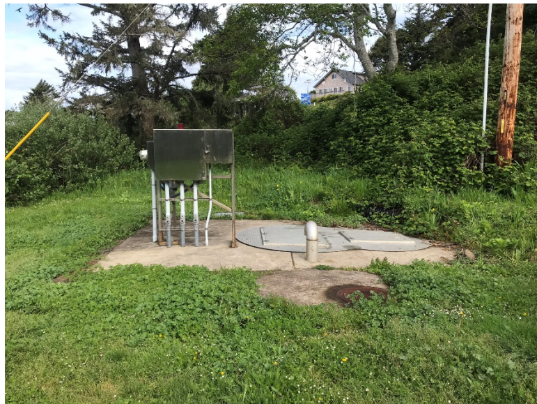
Figure 4-7 Riverside Pump Station
