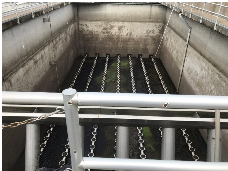
Figure 4-16 SBR Aeration Grid
