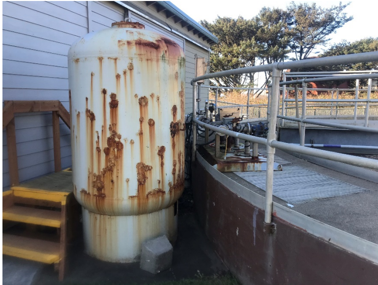
Figure 4-23 Non-Potable Water Pump Skid and Pressure Tank
