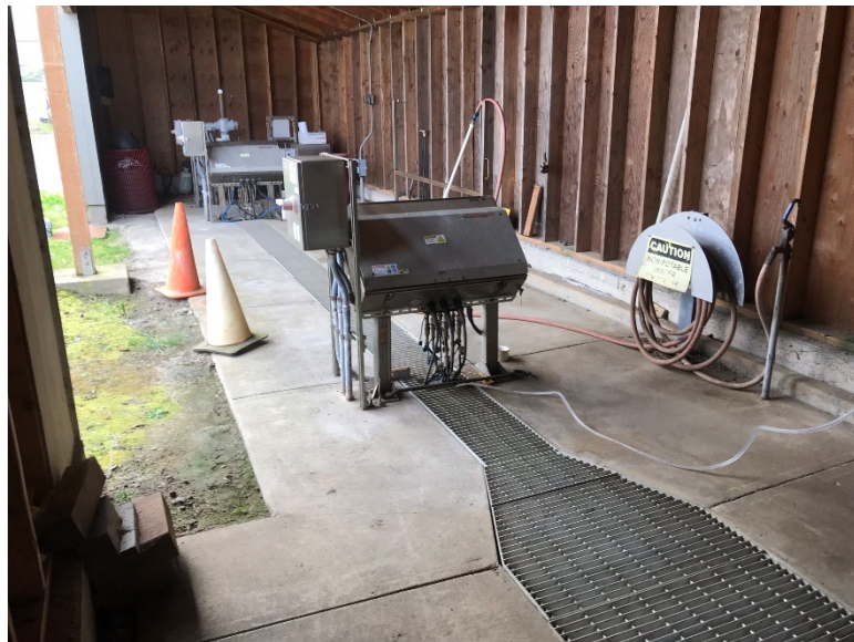
Figure 4-18 UV Disinfection System
