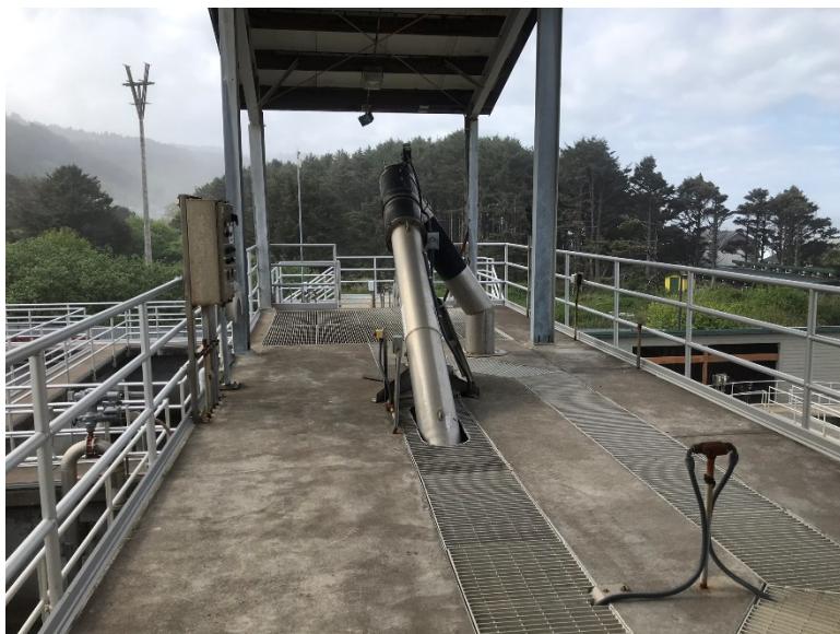
Figure 4-12 Headworks Fine Screen with Grit Removal Chamber
