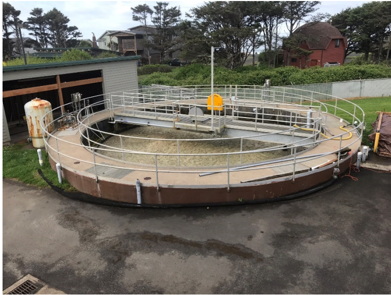
Figure 4-21 Sludge Storage Tank
