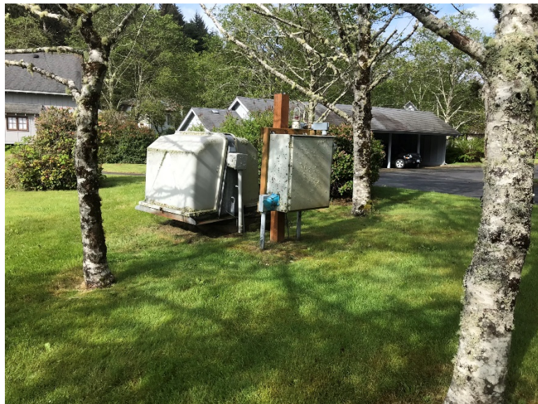
Figure 4-9 Quiet Water Pump Station
