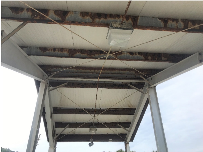
Figure 4-14 Headworks Shelter Corrosion
