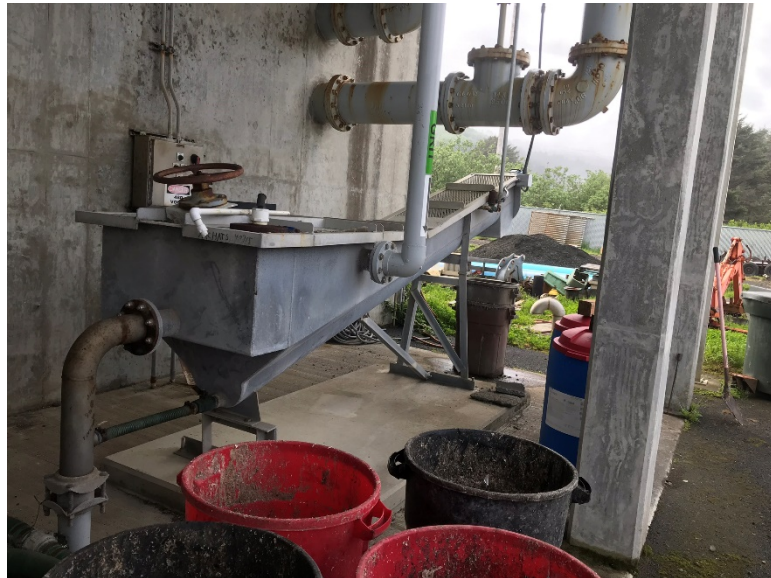
Figure 4-13 Headworks Grit Dewatering Equipment
