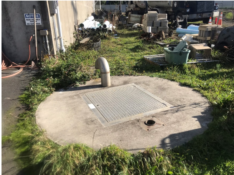
Figure 4-19 Drain Pump Station Wet Well
