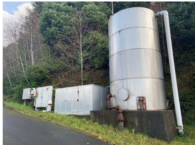
Figure 4-14 | 10,000 Gallon Middle Blackstone Reservoir & Pump Station
