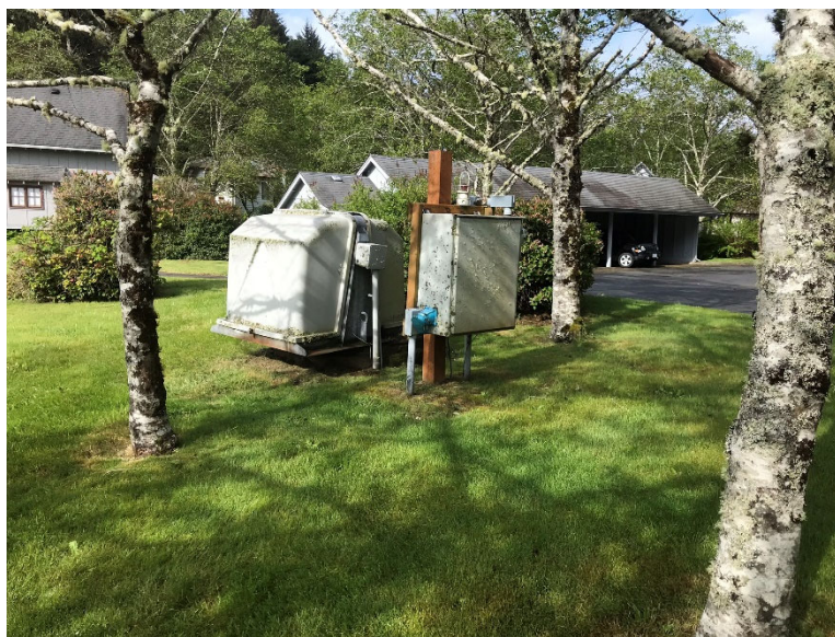
Figure 4-9 | Quiet Water Pump Station
