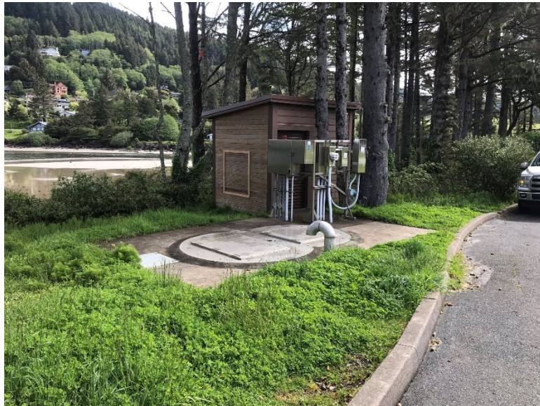
Figure 4-6 | Parkside Pump Station
