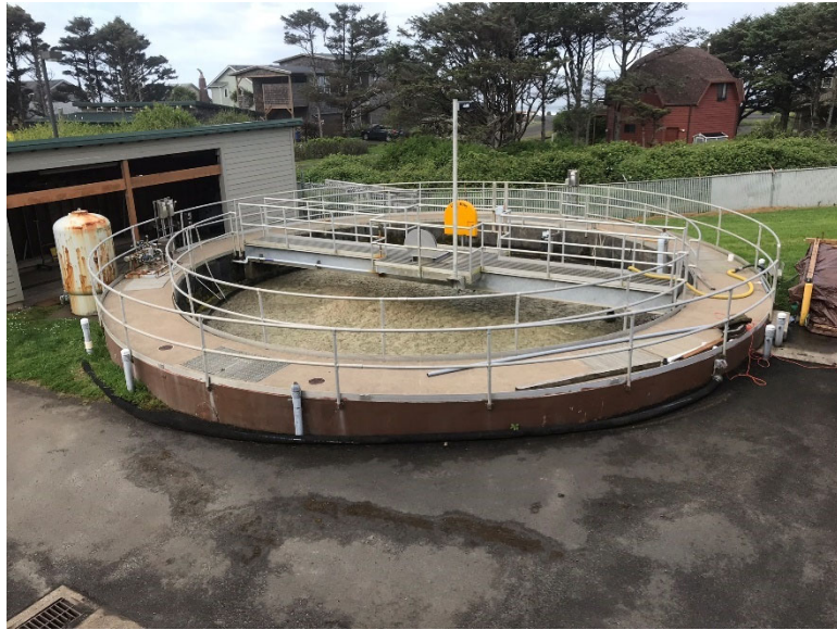
Figure 4-21 | Sludge Storage Tank
