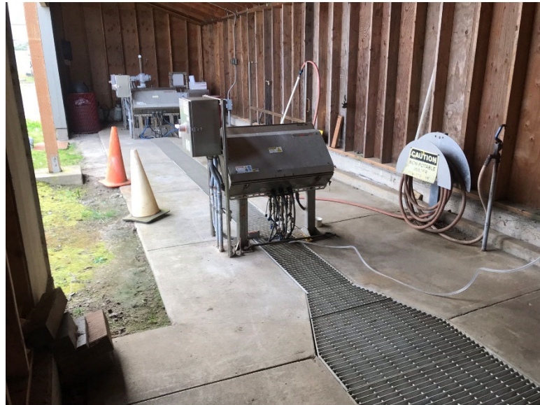
Figure 4-18 | UV Disinfection System
