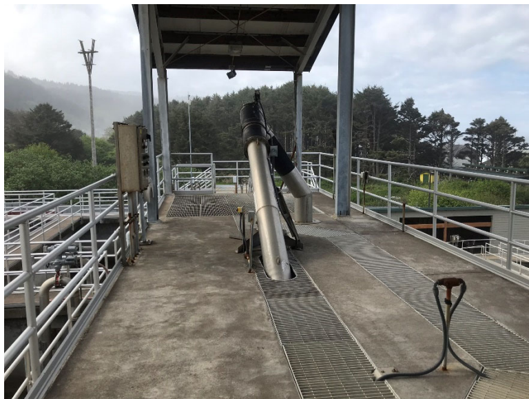
Figure 4-12 | Headworks Fine Screen with Grit Removal Chamber Behind
