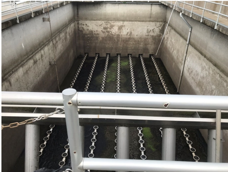
Figure 4-16 | SBR Aeration Grid
