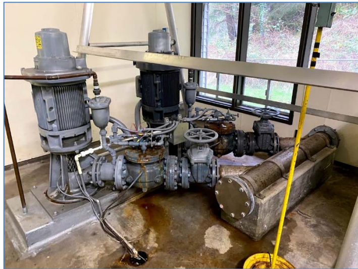
Figure 4-9 | High Service Pumps
