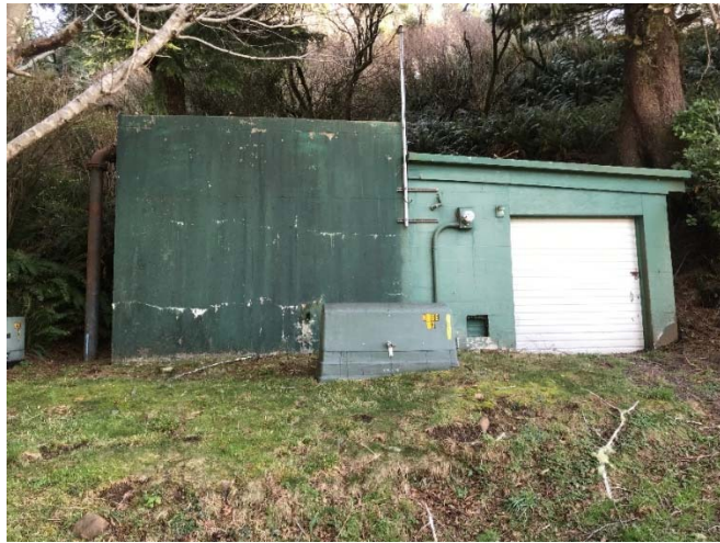
Figure 4-12 | 10,000 Gallon Horizon Hill Reservoir & Pump Station
