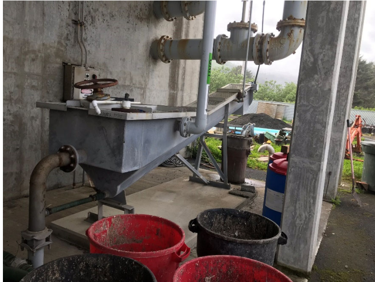
Figure 4-13 | Headworks Grit Dewatering Equipment
