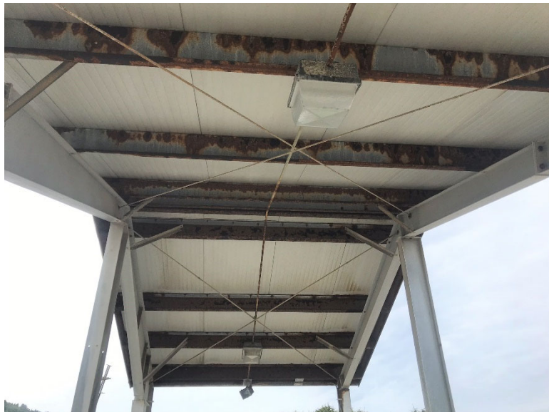
Figure 4-14 | Headworks Shelter Corrosion
