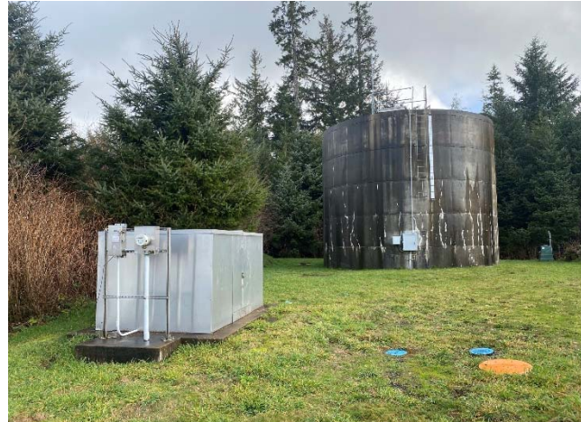
Figure 4-15 | 120,000 Gallon Upper Blackstone Reservoir and Pump Station
