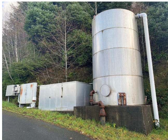
Figure 4-19 | Middle Blackstone Pump Station & Reservoir
