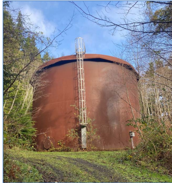
Figure 4-6 | Raw Water Storage Tank
