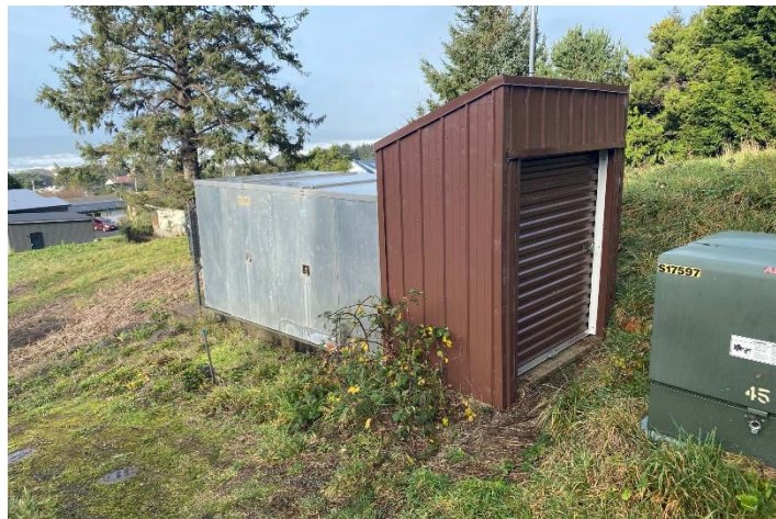
Figure 4-18 | Lower Blackstone Pump Station
