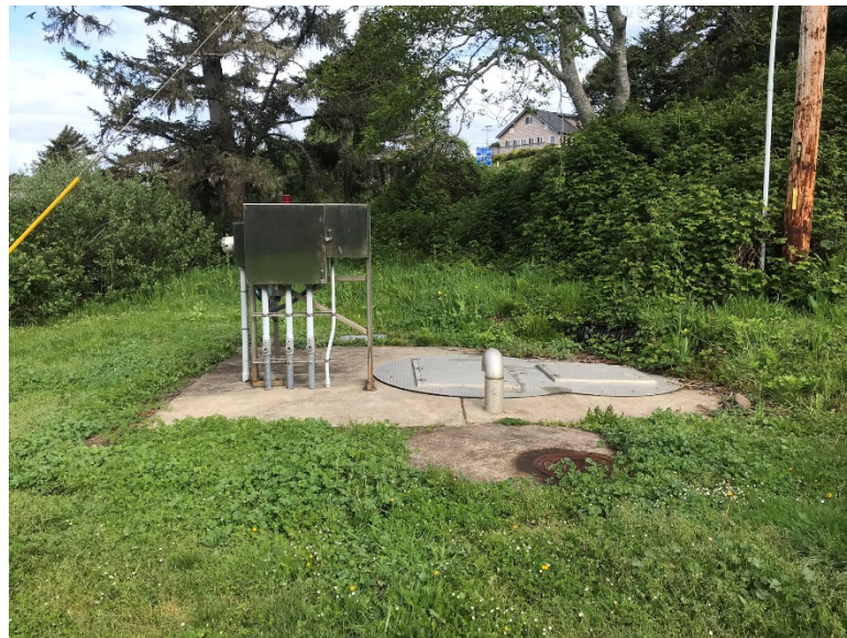
Figure 4-7 | Riverside Pump Station
