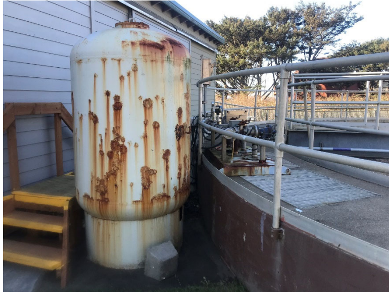
Figure 4-23 | Non-Potable Water Pump Skid and Pressure Tank
