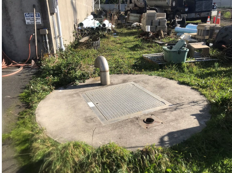
Figure 4-19 | Drain Pump Station Wet Well
