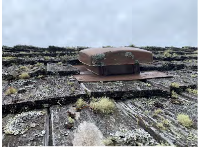
Figure 13- LICHEN AND MOSS ON MUSEUM ROOF
