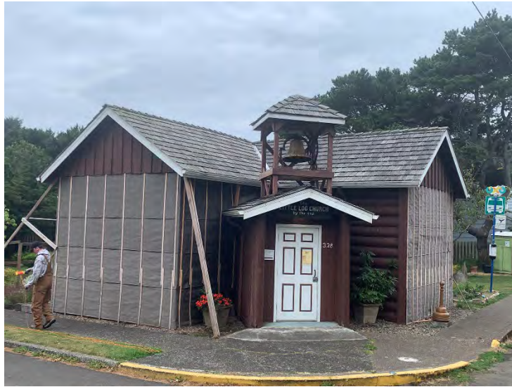
Figure 18 - CHURCH STRUCTURE EAST SIDE BRACING
