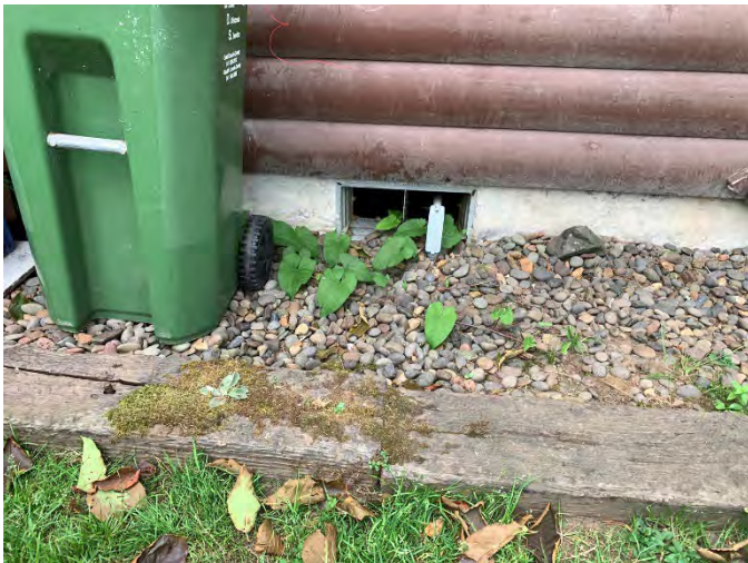
Figure 25 - CRAWL SPACE SCREEN MISSING
