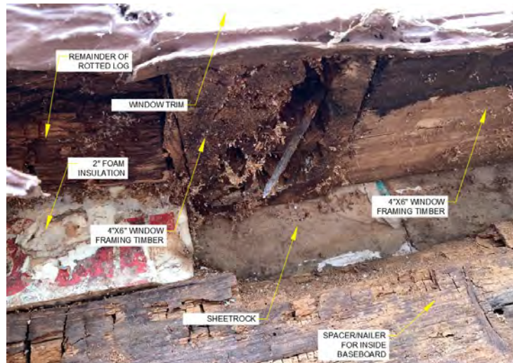
Figure 19 - ROT BELOW CHURCH WINDOW - LOOKING UP
