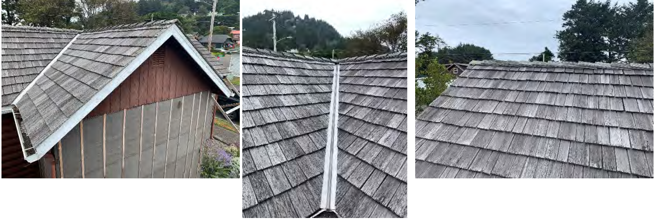
Figure 10- CHURCH CEDAR SHAKE ROOF
