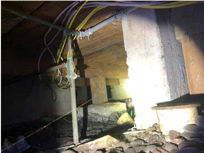
Figure 23- MIXED METAL PLUMBING CONNECTION - COPPER TO GALVANIZED
