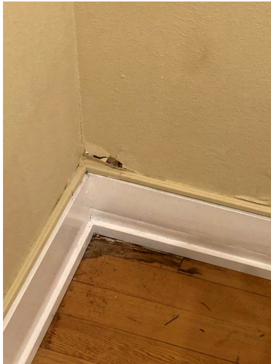
Figure 21 - WATER DAMAGE - SOUTHEAST CORNER
