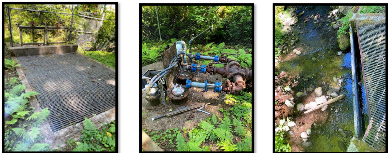
FIGURE 2.6 – VINGIE CREEK INTAKE AND PUMP PLUMBING
