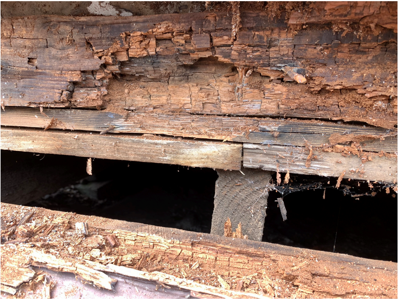
Decay of Log Siding at Main Floor Level
