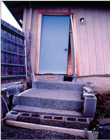
House cracks. Photo credit: Scott Burns.
