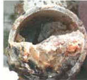
Grease clog inside a pipe.
